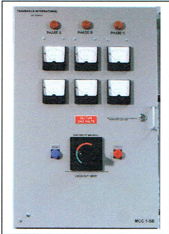
3-phase Power Switchboard • voltage & current instrumentation • 3-phase line monitor & failure relay • main circuit breaker • lock/tagout interlock on cabinet
